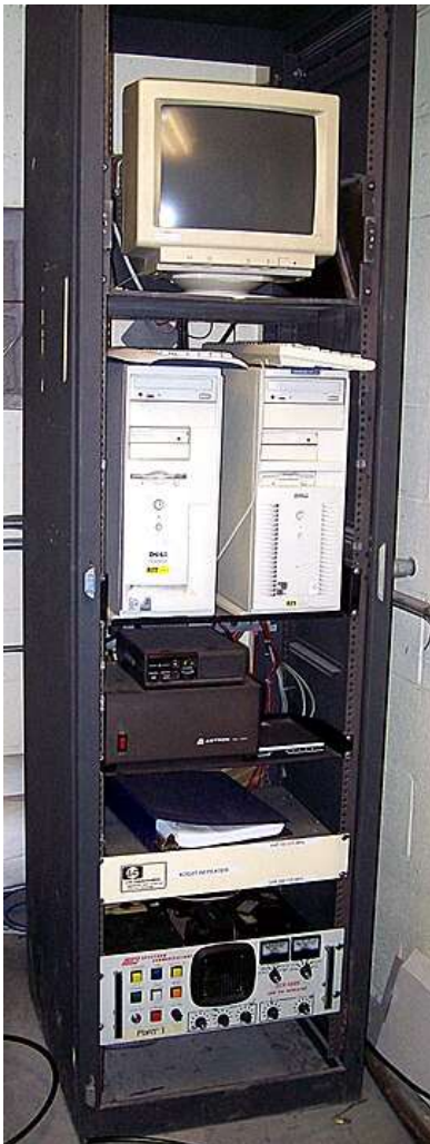
70 cms repeater cabinet - 1*
